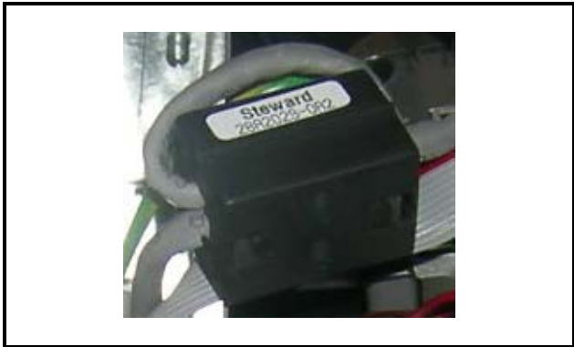
Figure 2-2 - Ferrite Installation on Ethernet Cable
