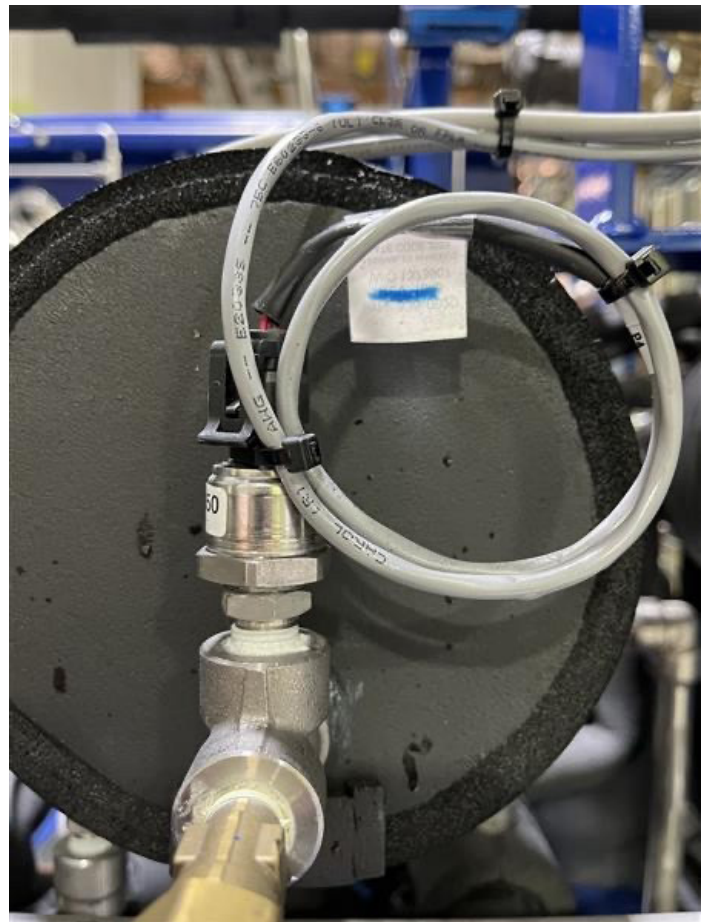
Transducer Cable Harness
