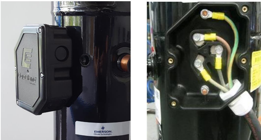
Figure 22: Terminal box IP54 and correct electrical installation with cable gland
