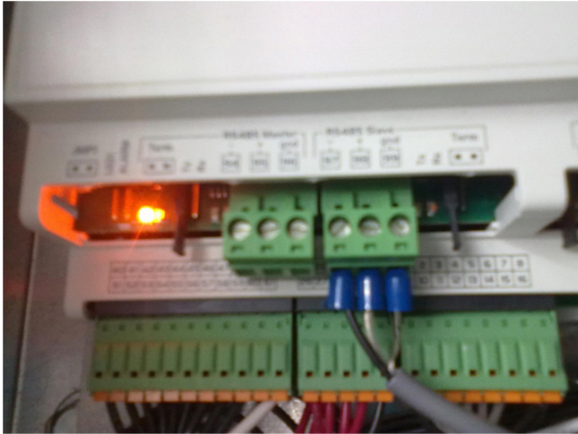
Multi-Zone Leak Detector Wiring
