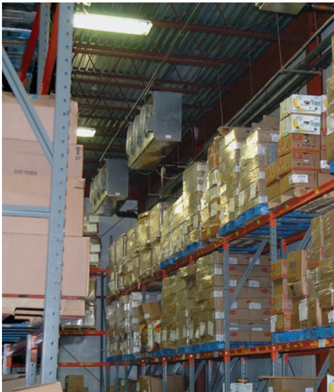
Meeting the food bank's cold storage requirements had become increasingly difficult for the facility's legacy, fixed-capacity refrigeration system.
