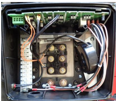
Figure 3: Copeland Compressor Electronics module cover open
