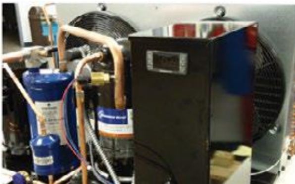
Figure 11 Large Black Electrical Box
