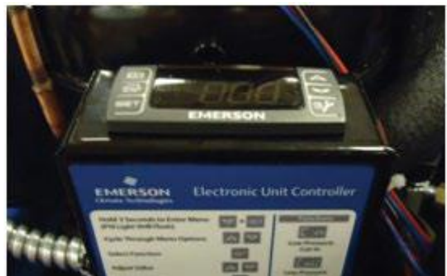
Figure 10 Small Black Electrical Box
