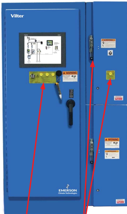
Main power circuit voltage indicator
