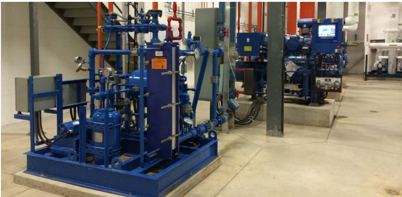
Figure 5: Vilter ammonia heat pump installation at a pork processing facility
