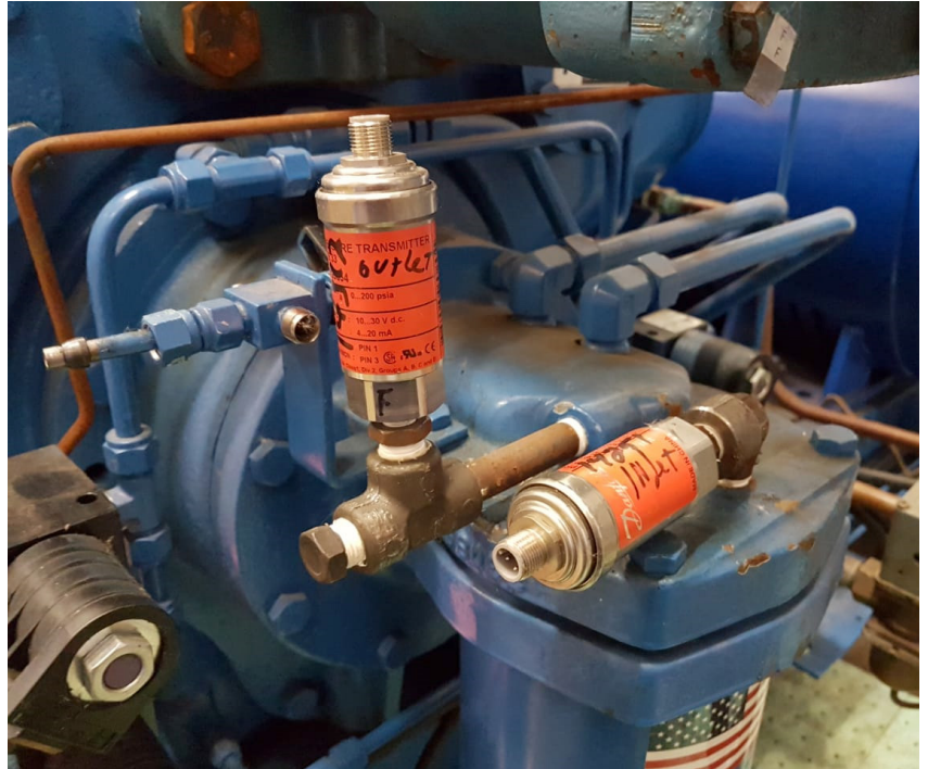
Figure 12. Tri-Micro Filter with Pressure Transducers for Inlet and Outlet Pressures
