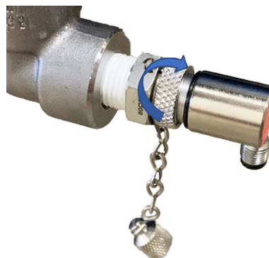
Figure 5-4(b) Valve Shown Ready for Oil Sampling
