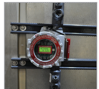
Enclosure Gas Detection
