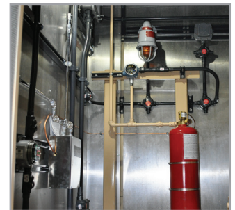
Fire Suppression System
