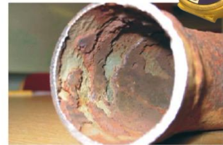
Pipe corrosion caused by carbonic acid
